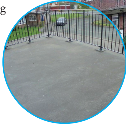
Brindley Asphalt Roofing applied the IKO Permaphalt mastic asphalt system for the Merridale Court project
