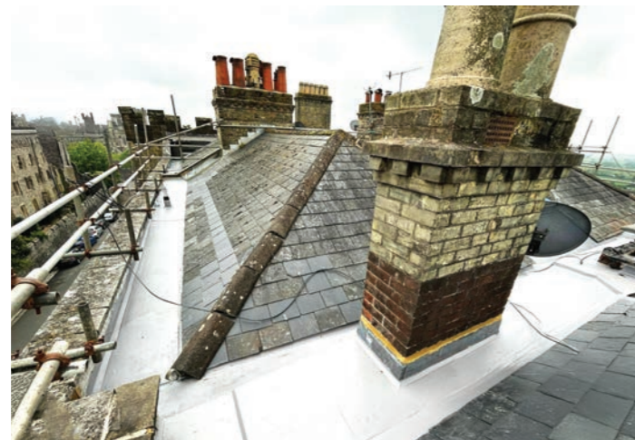
This project involved a significant amount of asphalt heritage detailing - in fact much more than the flat roofing area.
